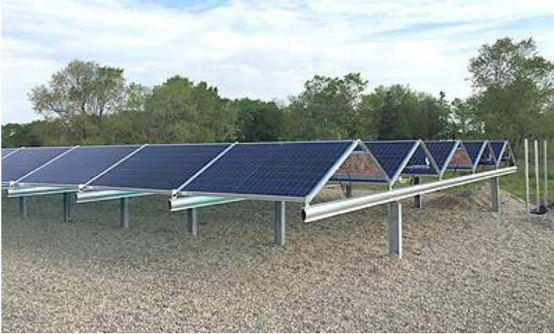
Runestone Electric Association's 44 KW Community Solar Alexandria, MN
