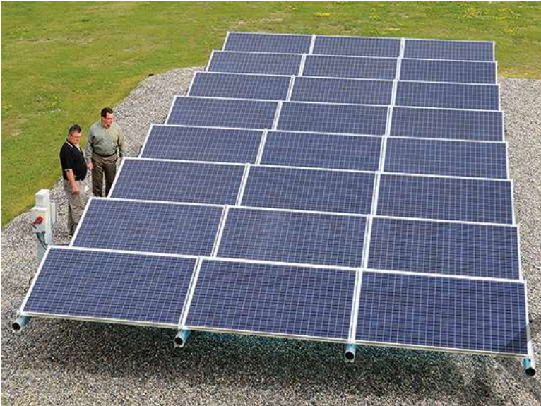
Roseau Electric Cooperative's 10 kW Demonstration Solar System Roseau, MN
