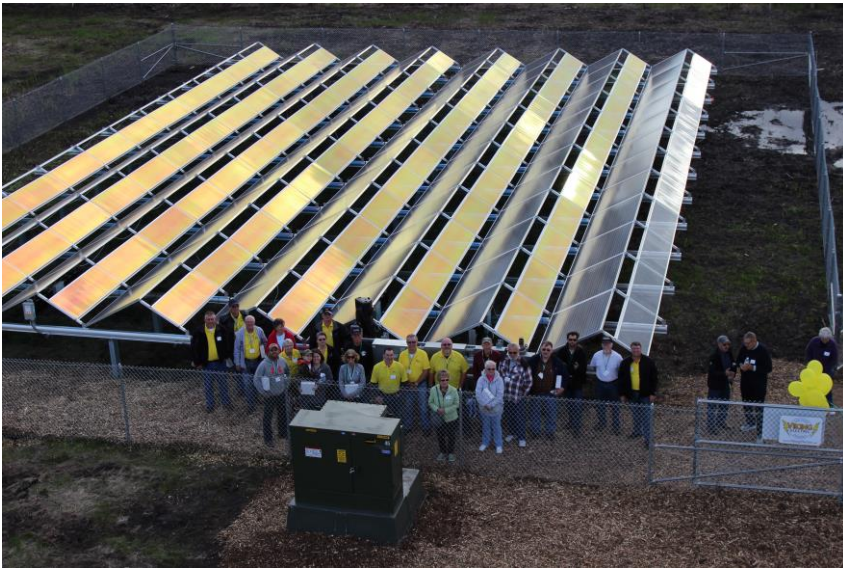
Meeker Cooperative's 39.36 kW(DC) Member Solar System Litchfield, MN
